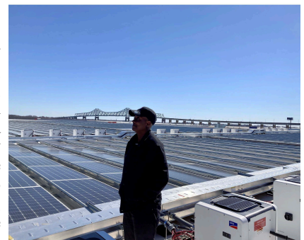
Joelle on site at NJ's first community solar project in Perth Amboy
